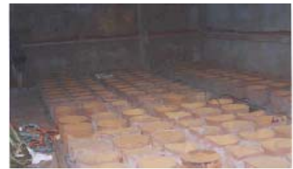
Condition of Old Floors & Thimbles
